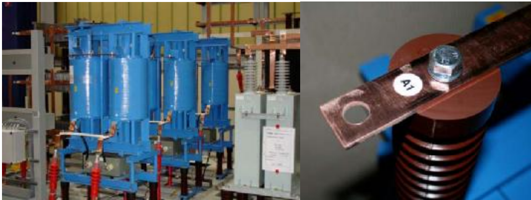
Figure 20: Examples for connected product on standoff insulators (left) and marking of terminal on top of core (right)
